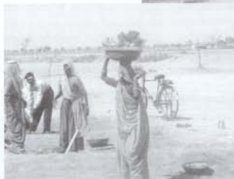
Women contributing to the construction of an anicut and pond to recharge depleting ground water in Lawadi, Rajasthan.
