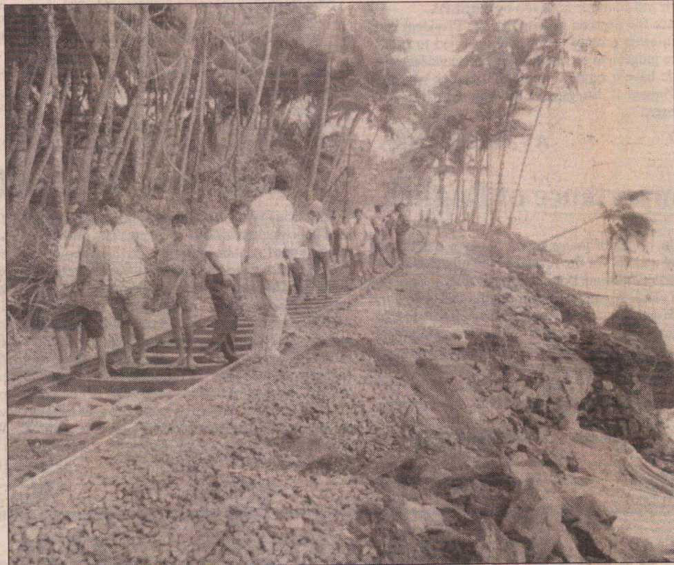
Sea eroding into the railway line
