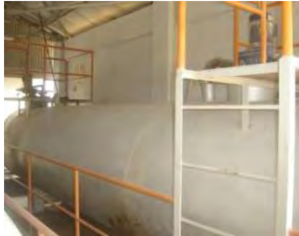
Intermediate Tank (Day Tank)
