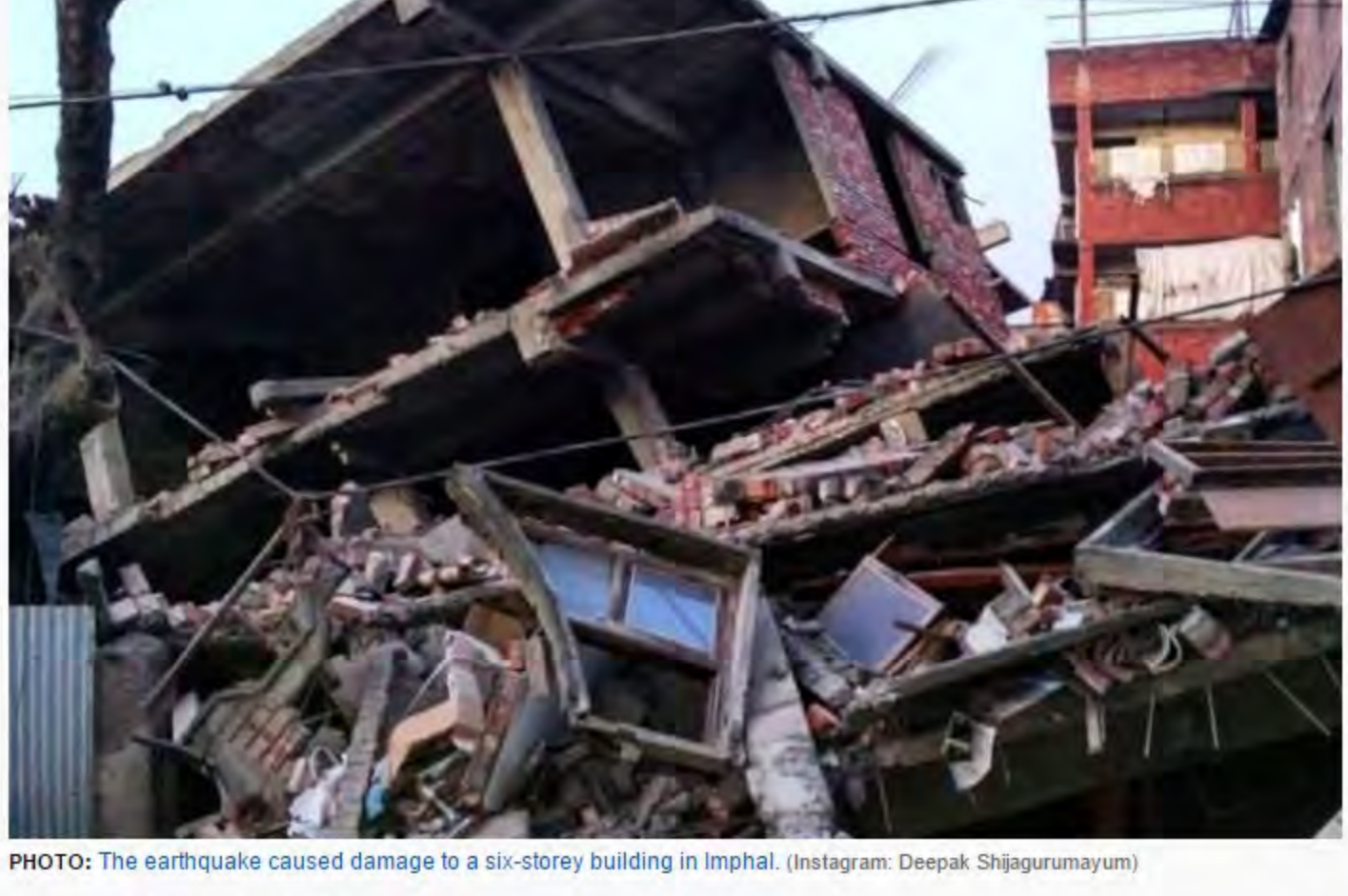
PHOTO: The earthquake caused damage to a six-storey building in Imphal. (Instagram: Deepak Shigajurumayum)
