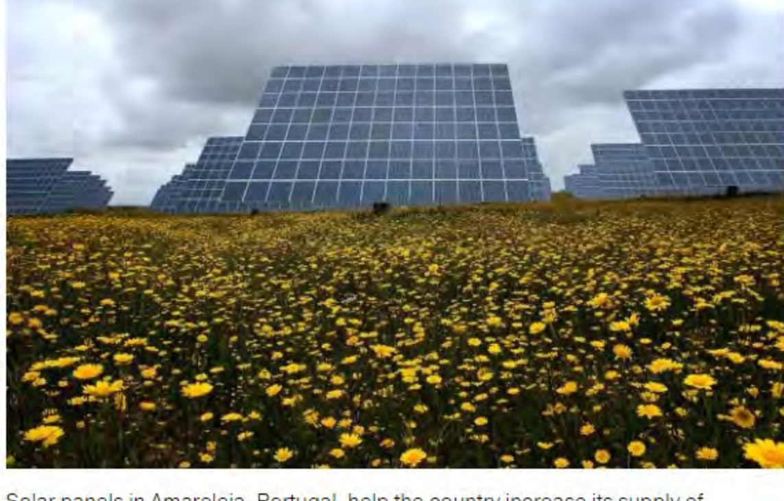
Solar panels in Amareleja, Portugal, help the country increase its supply of renewable energy.
