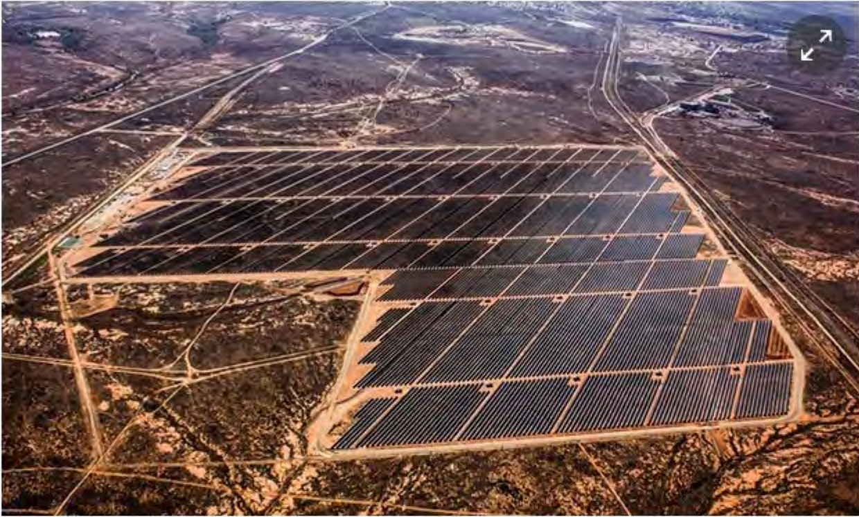
The recently completed Broken Hill solar plant – one of the largest in Australia. Solar power accounts for almost 60% of employment in renewable energy. Photograph: Australian Renewable Energy Agency
