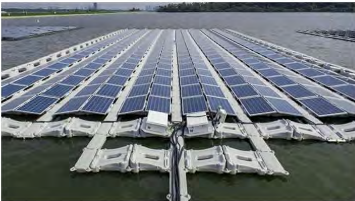
A one-megawatt floating solar test project in Singapore.
