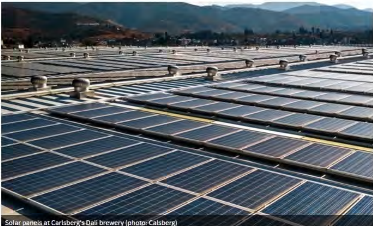
Solar panels at Carlsberg's Dali brewery (photo: Calsberg)
